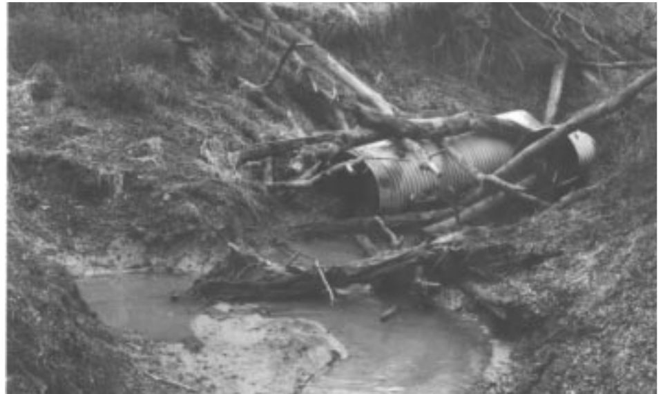
Unkempt drainage system.
